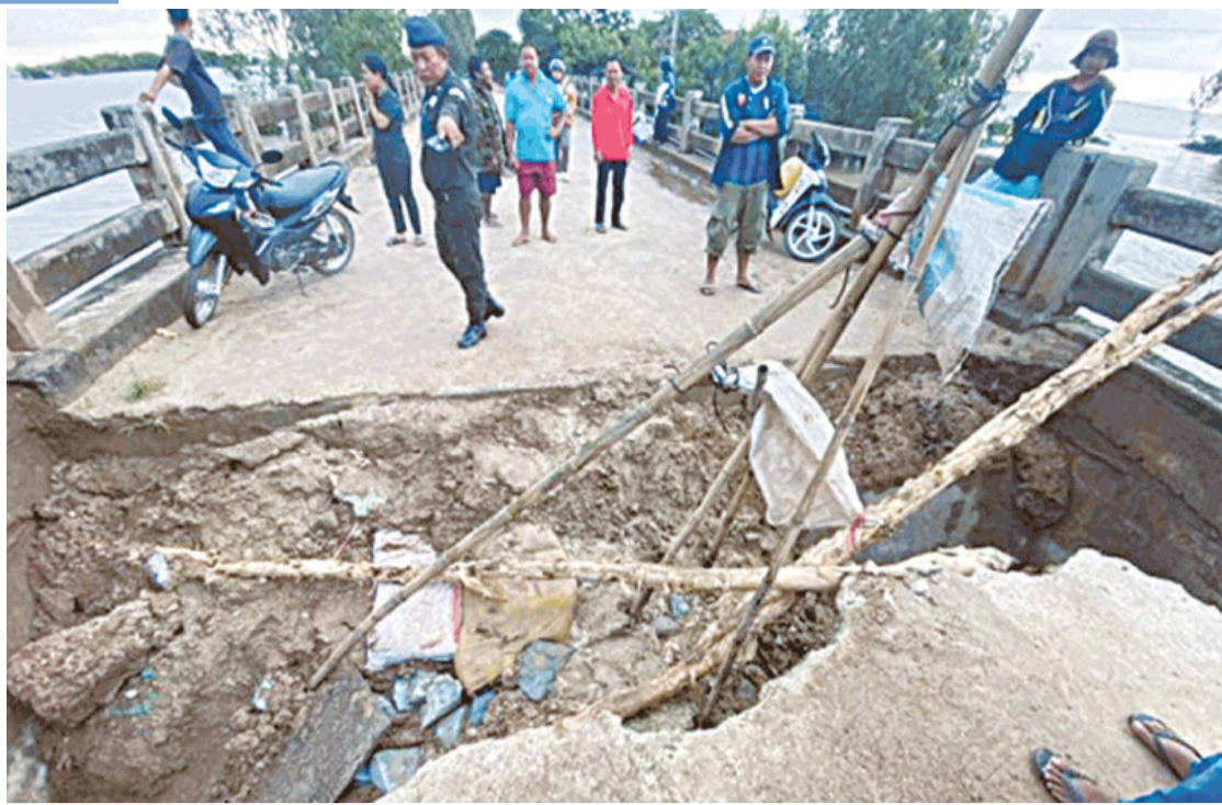
A bridge damaged by floodwaters.—Courtesy The Phnom Penh Post
