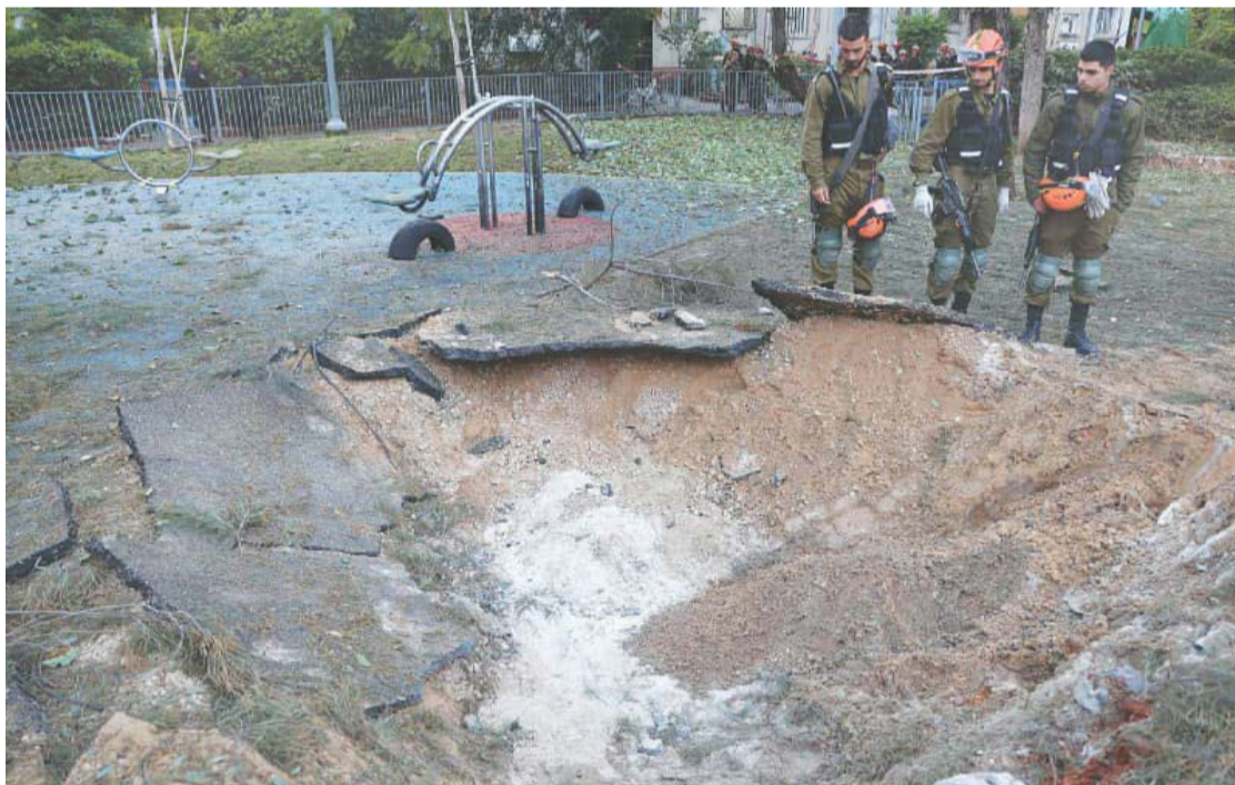
Tel Aviv: Israeli emergency responders inspect a crater at the site where a projectile fired from Yemen landed, on Saturday.
