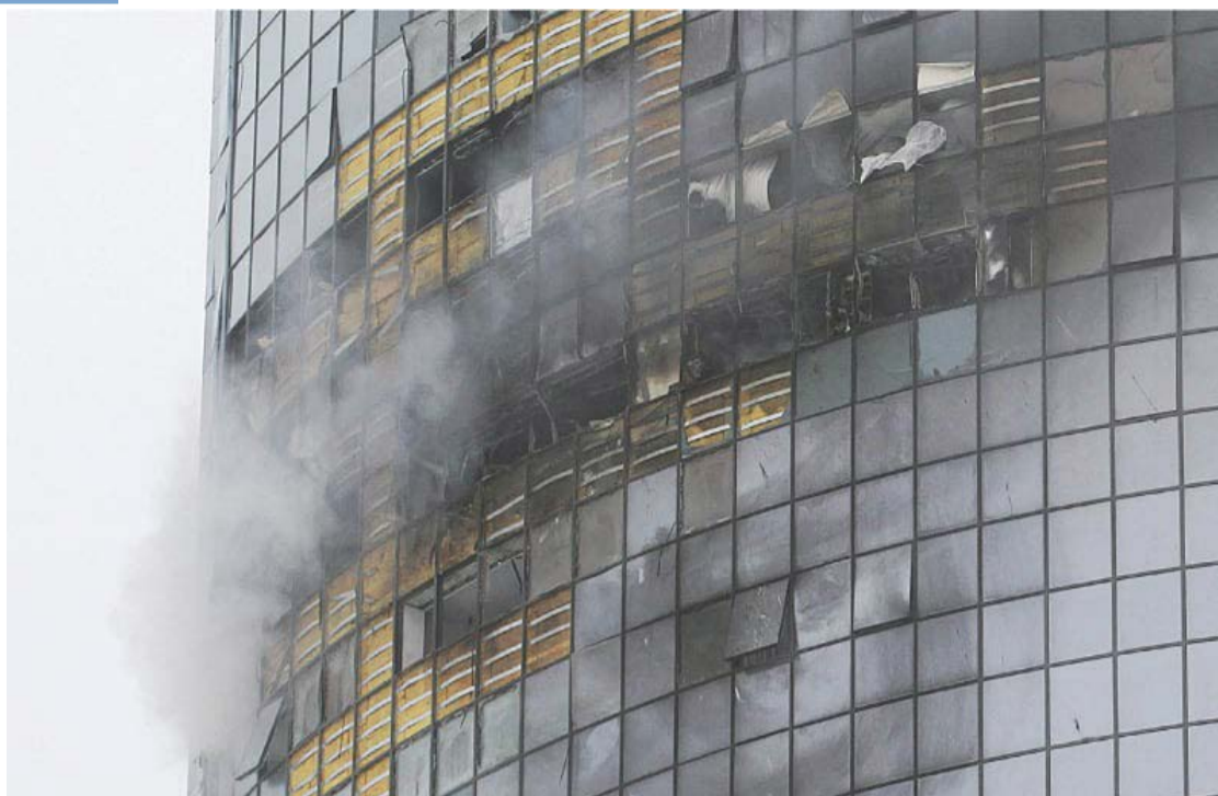
A VIEW of a damaged multi-storey residential building in Kazan, Russia, following a Ukrainian drone attack.—
