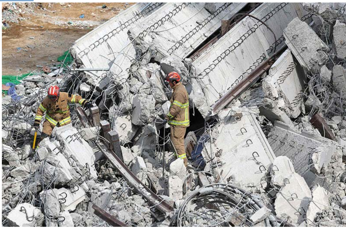
Rescuers search for missing workers after a bridge collapsed at an expressway construction site in Anseong on February 25
